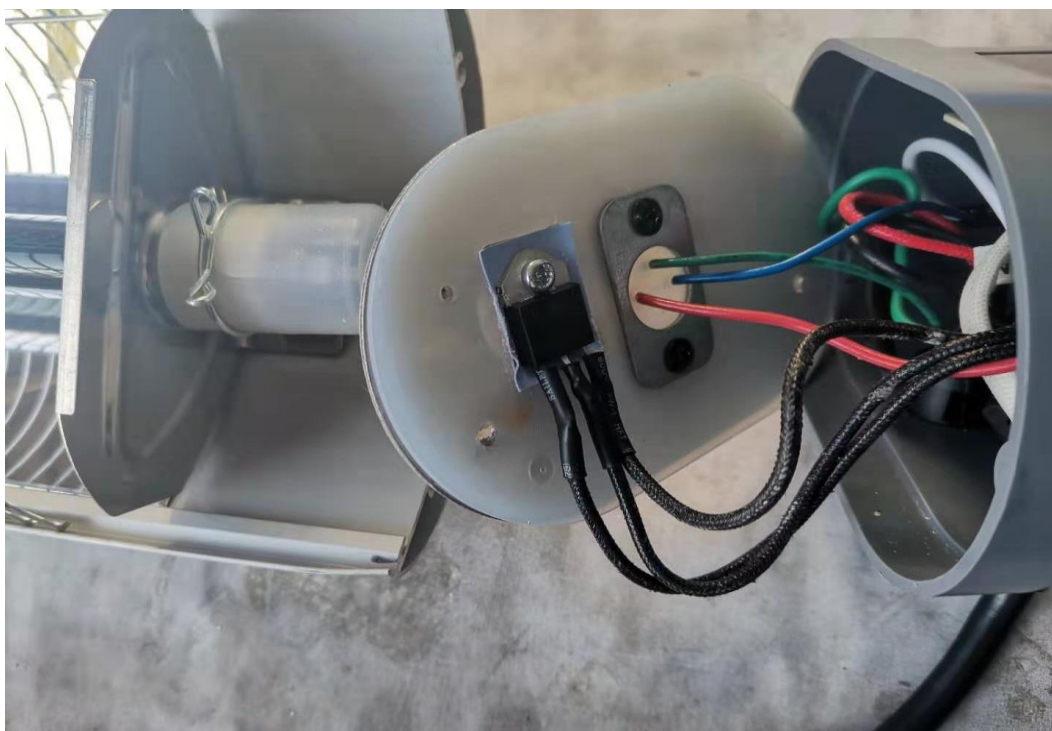
Photo 19A - Alternative internal view of PHF-1500R
